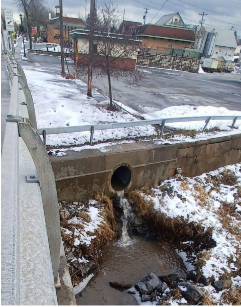
Figure 6: A photograph of the stormwater outfall under the Main Street bridge in Canton, NY.
