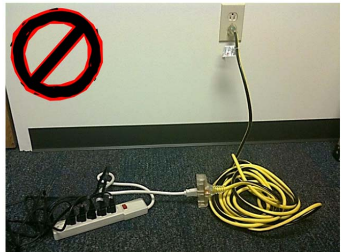
Improper power strip use; plugged into extension cord. Power strips must be plugged directly into an outlet, and extension cords are for short term use only.
