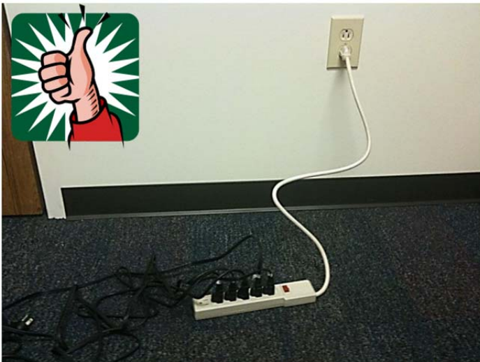
Proper use of power strip, plugged directly into a wall outlet.
