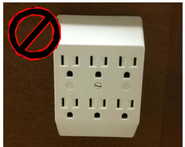
Prohibited multi-outlet adapter; multi-outlet adapters must have resettable circuit breakers.
